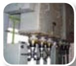
Power sensitive equipment
